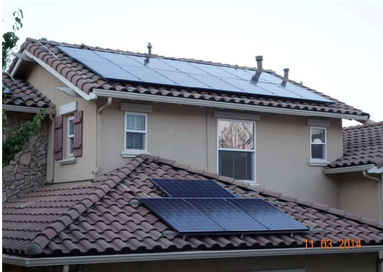
Solar system on tile roof
