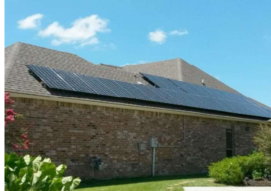
Solar system on composite shingle roof
